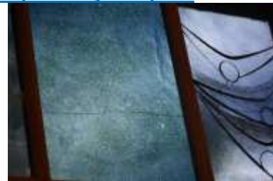
repair windows with cracked glass
