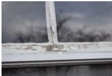
New putty required throughout
